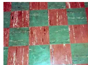
9"x9" Asbestos-Containing Floor Tile
