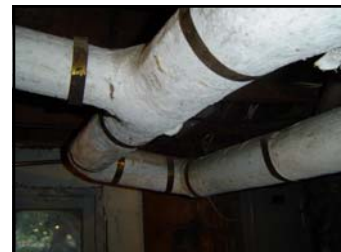
Asbestos-Containing Pipe Insulation
