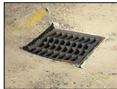
Parking Lot Storm Drain
